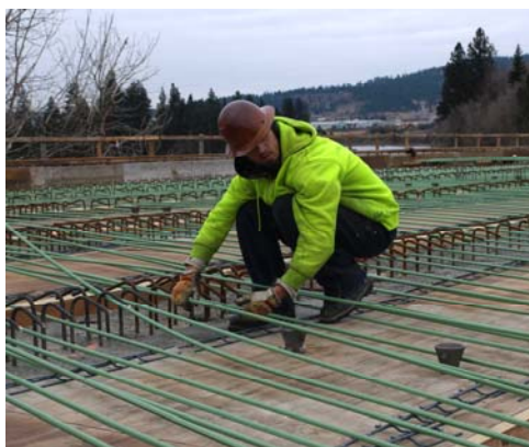
Hundreds of pieces of specially treated rebar will provide reinforcement to the concrete decking.
