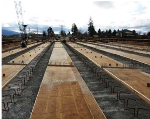
Concrete forms placed between the girders will provide support during the pouring of the concrete decking (driving surface). Once the concrete has cured, these plywood forms will be removed.
