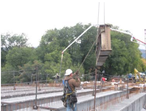
A bridge worker guides a giant section of the temporary work pier up and away from the newly placed girders.
