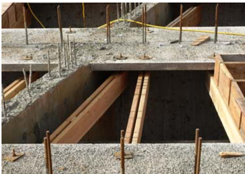
Shown to the left of two wood cross braces, above, a concrete diaphragm helps stabilize the bridge structure.
